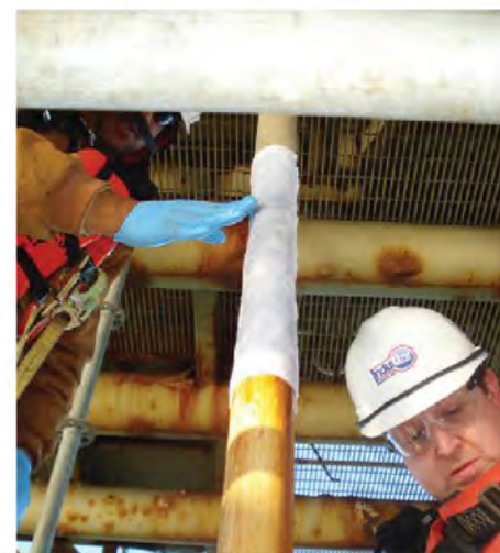
InduMar's Bill Nobles supervises the application of the STOP IT® Pipe Repair System.
